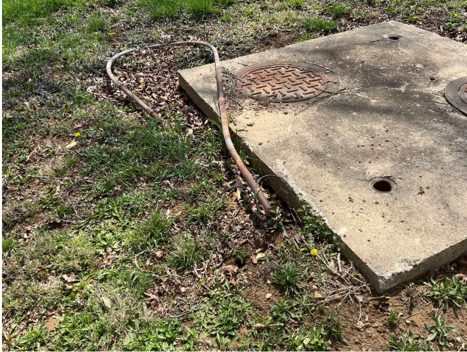
Figure 35: View of exposed electrical area on site.
