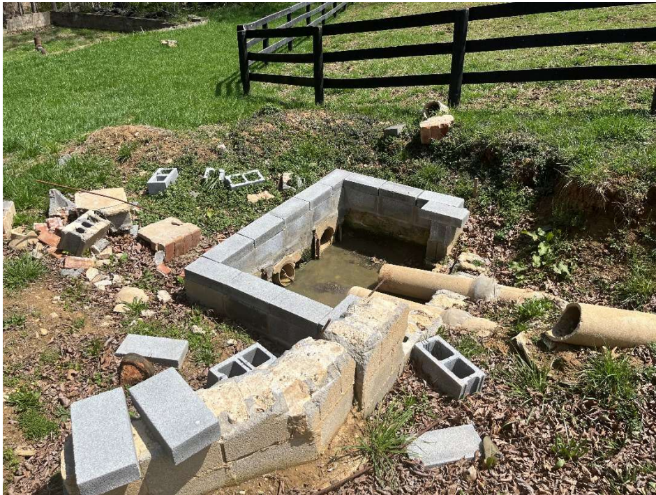
Figure 22: View of septic system drain to secondary sand filtration
