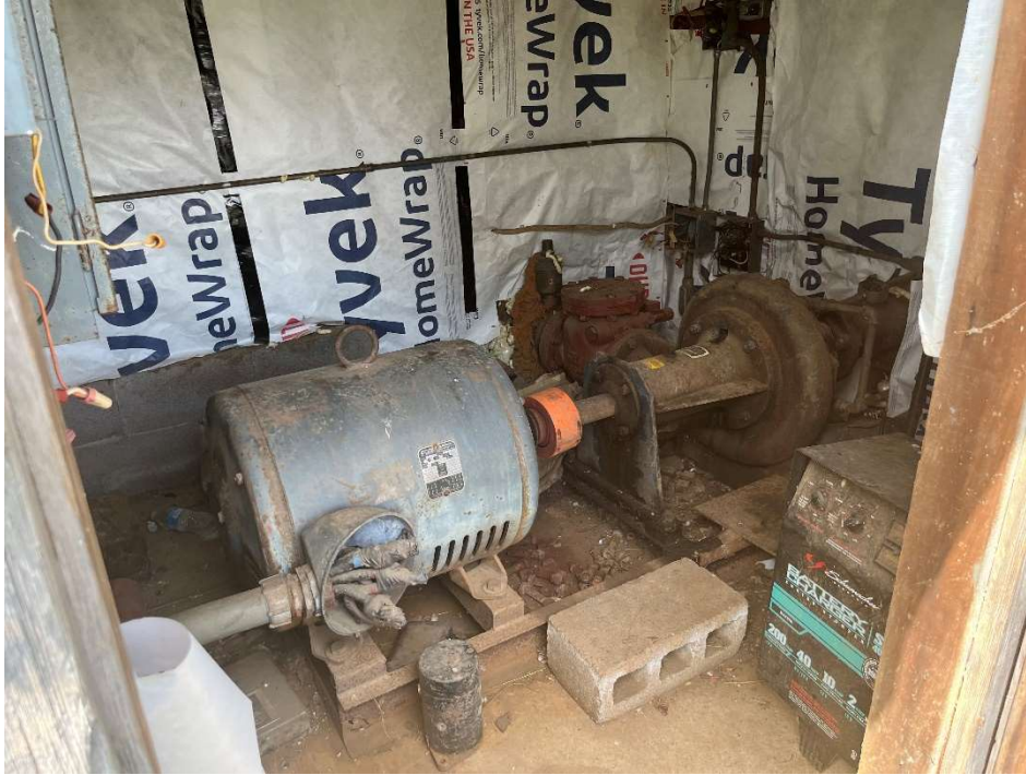
Figure 45: Inside view of the new pump house.
