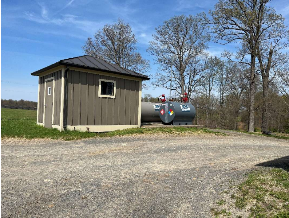
Figure 109: View of the on-site storage tanks.
