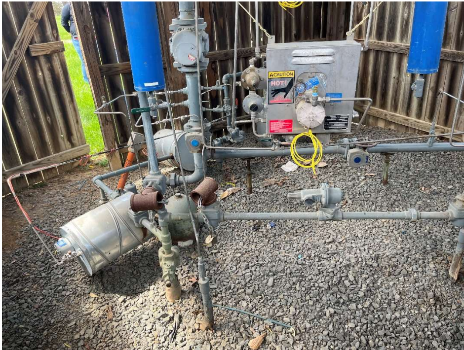
Figure 96: Close up view of the mechanics for the Columbia pipeline.
