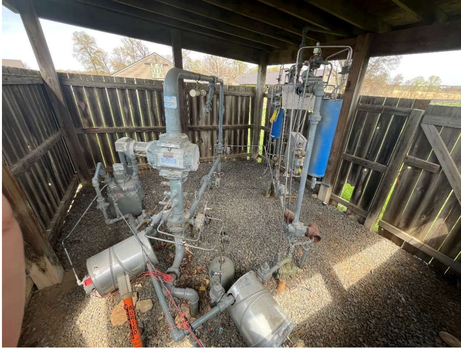
Figure 95 View of inside the Columbia pipeline area.
