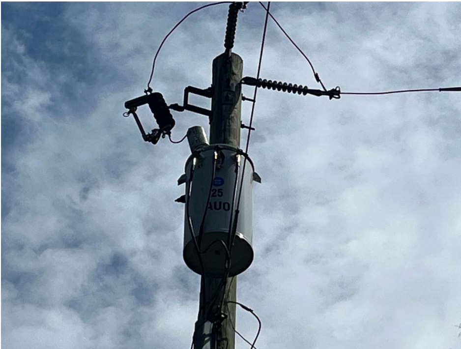
Figure 102: View of the electrical transformer, a sticker on the transformer says, "No PCBs".
