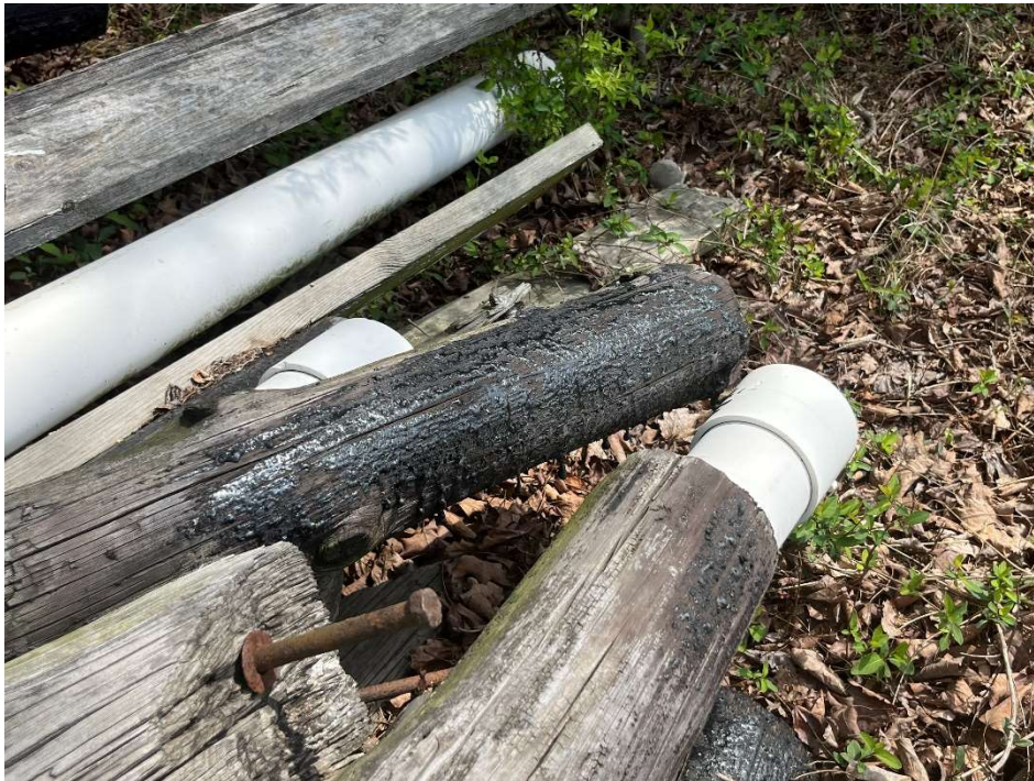
Figure 72: Zoomed in view of the ends of electrical poles. It appears a black substance is leaking off the poles.
