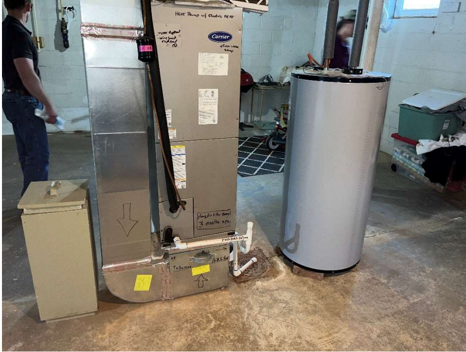
Figure 105: View of the water heater for the one site residence.
