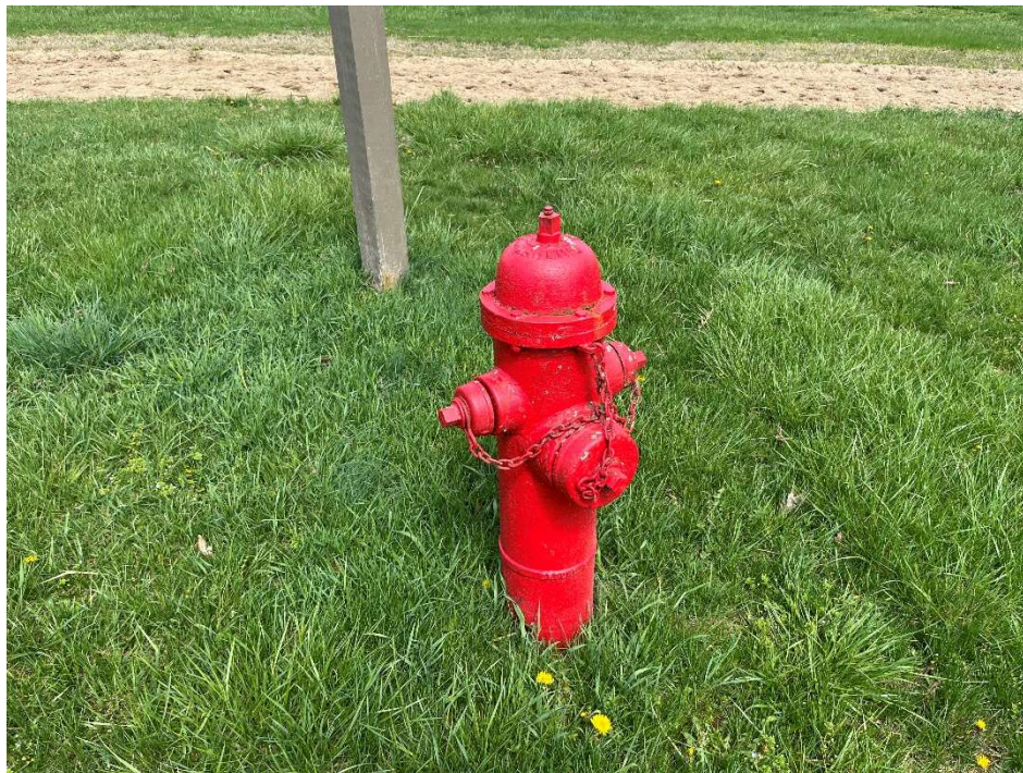
Figure 98: View of one of the fire hydrants on the Site.
