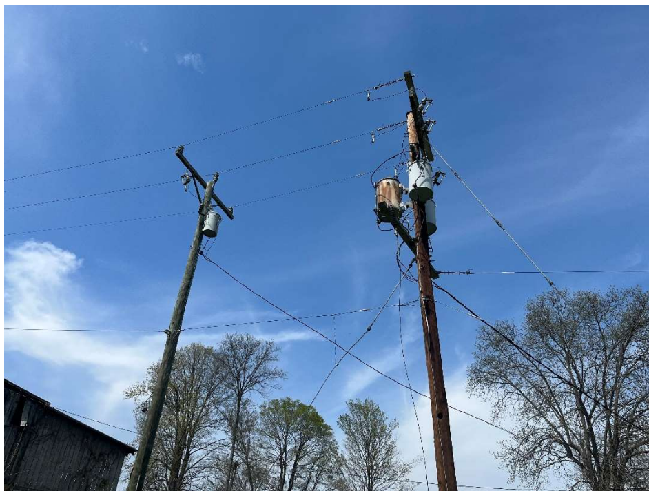
Figure 41: View of electrical transformers and lines located at the northern portion of the site.
