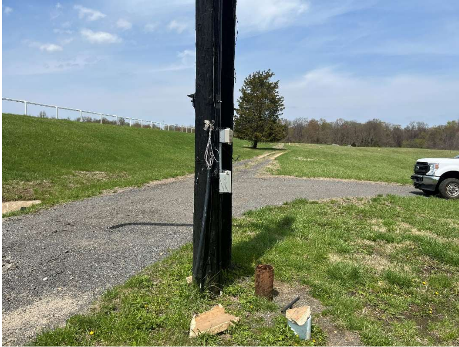
Figure 75: View of the exposed electrical wires under the faucet.
