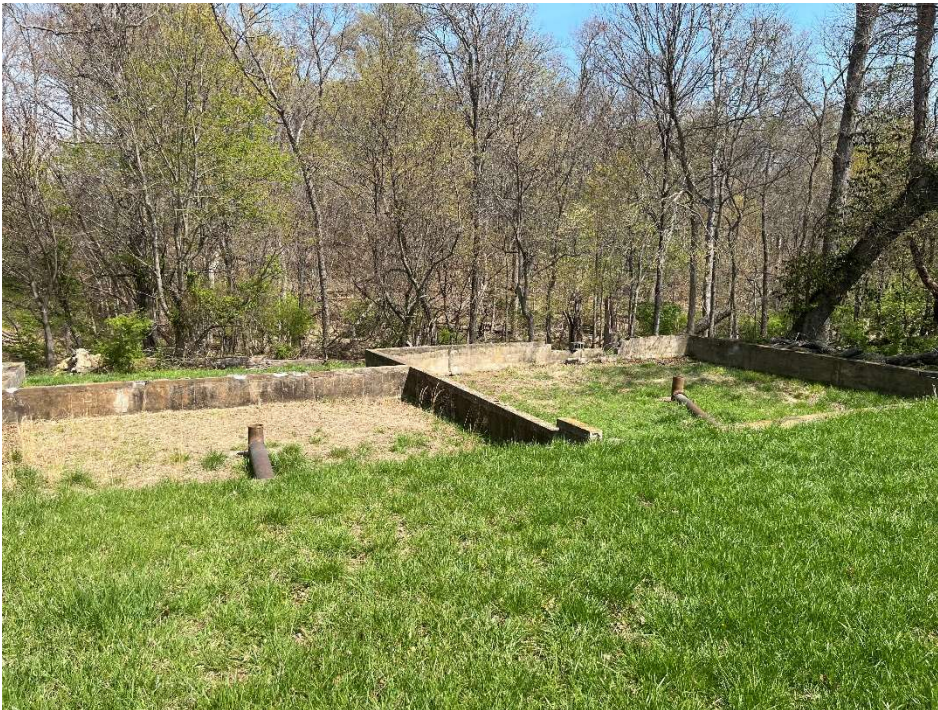
Figure 24: View of secondary sand filtration for septic system
