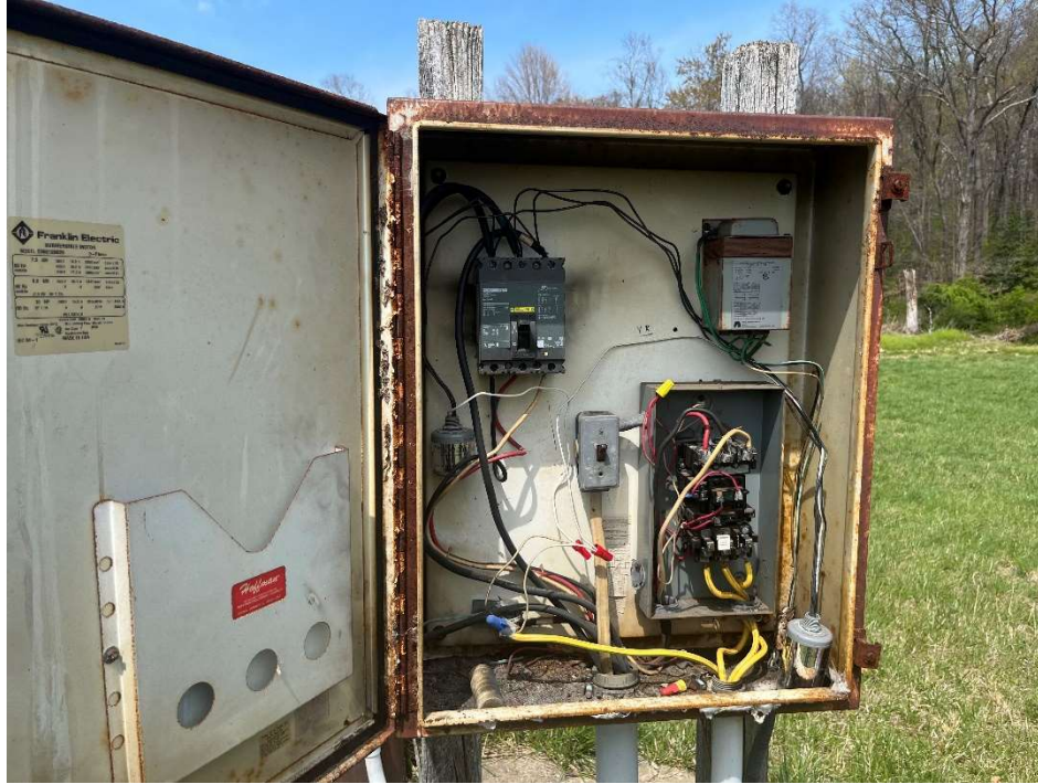
Figure 11: View of inside pump mechanics' box.
