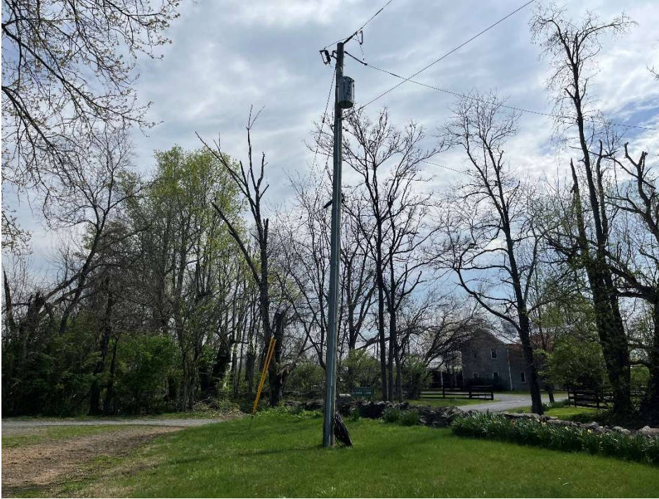
Figure 101: Zoomed out view of electrical pole by the on-site residences.
