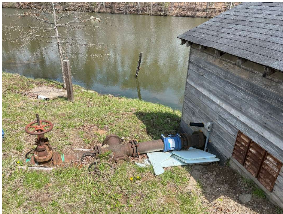
Figure 51: View of mechanics outside of pump house.
