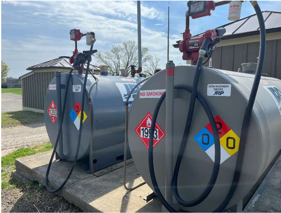
Figure 111: View of the onsite fuel tanks.
