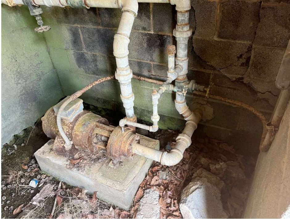
Figure 49: Close up view of older pump.
