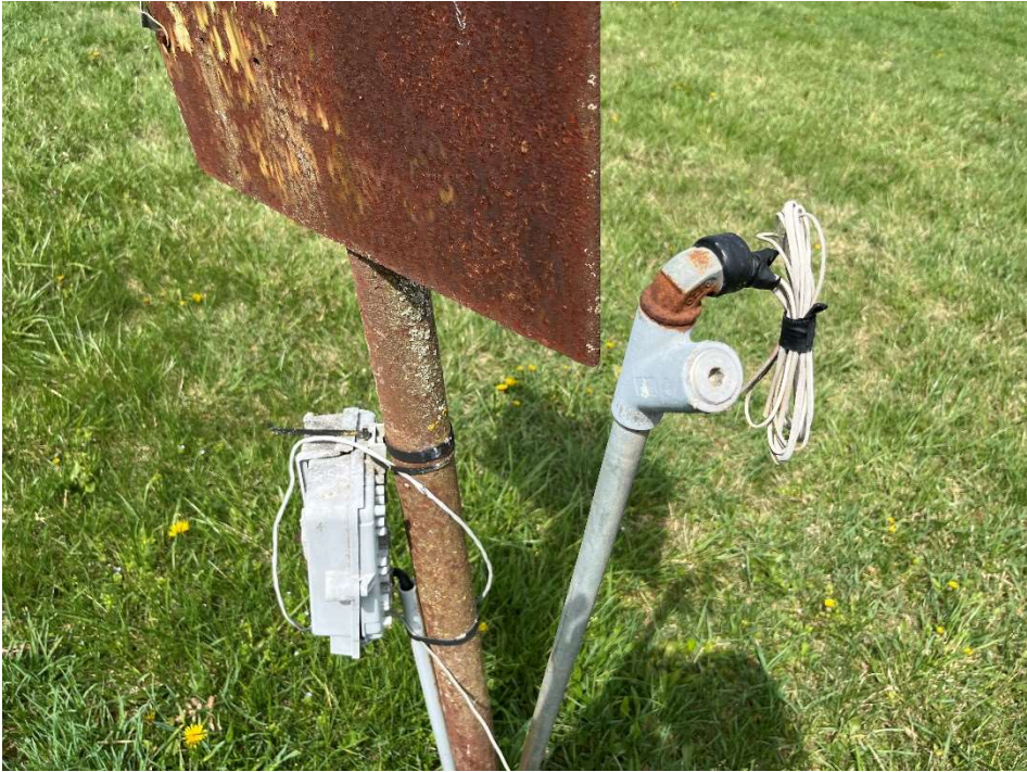
Figure 94: View of exposed electrical equipment around the eroded sign.
