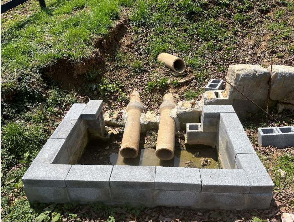
Figure 23: View of septic system drain to secondary sand filtration
